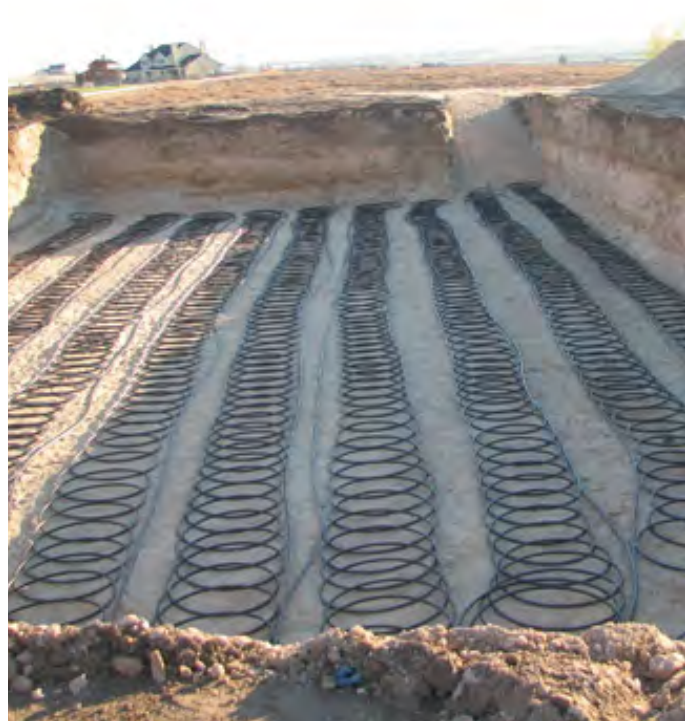
Geothermal Piping (located beneath open spaces)
