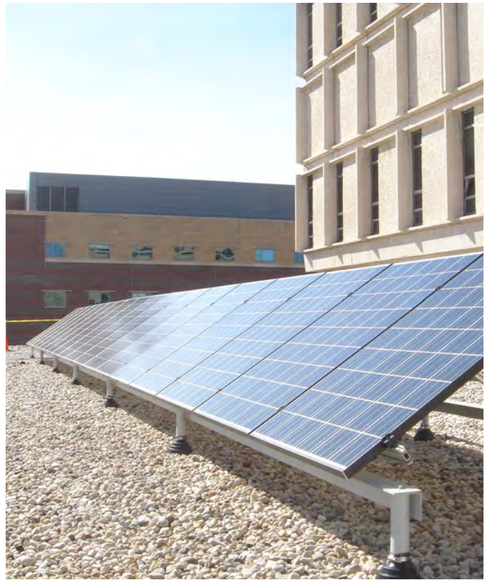
Peak Shaving - Photovoltaic Panels on Rooftops
